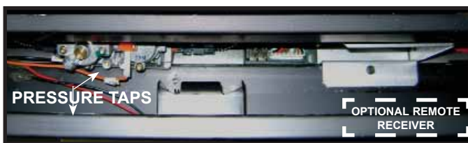
Figure 11.5 Valve Pressure Taps and Remote Receiver Location
